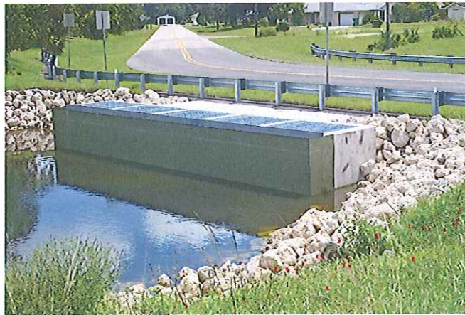
Newly constructed Water Control Structure #504 on Jupiter Waterway with fiberglass skimmer to prevent clogging and triple 72" concrete culvert pipes under Chancellor Blvd through a cooperative joint project with Charlotte County Public Works
