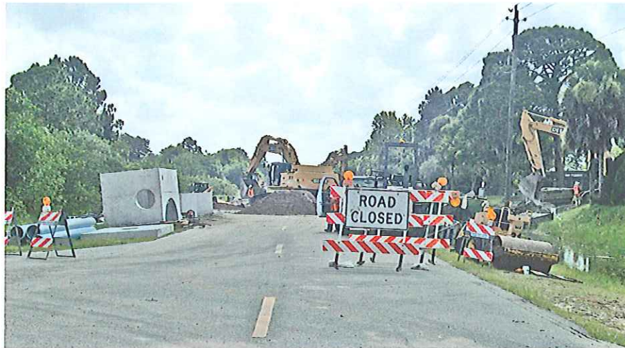
Water Control Structure #501 on Cheshire Waterway – Replacing concrete structure and 60” diameter corroded metal pipe with concrete pipe
