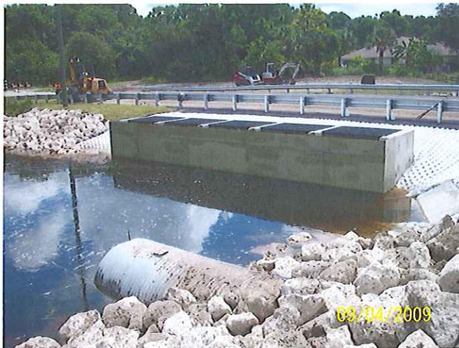
Newly constructed Water Control Structure #503 on Apollo Waterway with fiberglass skimmer to prevent clogging and triple 72" concrete culvert pipes under Chancellor Blvd through a cooperative joint project with Charlotte County Public Works
