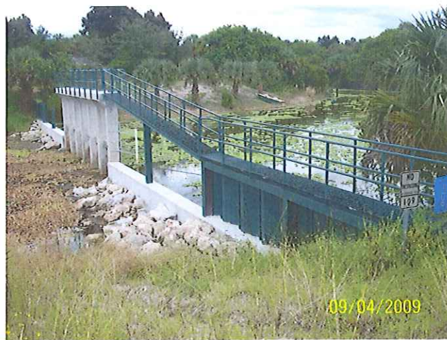
Newly retrofitted Water Control Structure #109 on Cocoplum Waterway with concrete weir and 6 new stainless steel gates
