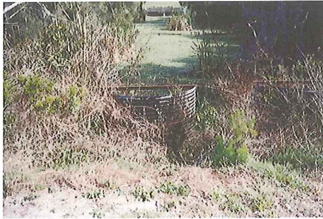
Old Water Control Structure #504 on Jupiter Waterway - Note corroded metal drop pipe design which is subject to clogging
