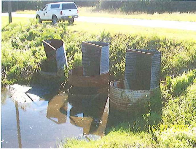
Old Water Control Structure #503 on Apollo Waterway - Note corroded metal drop pipe design which is subject to clogging
