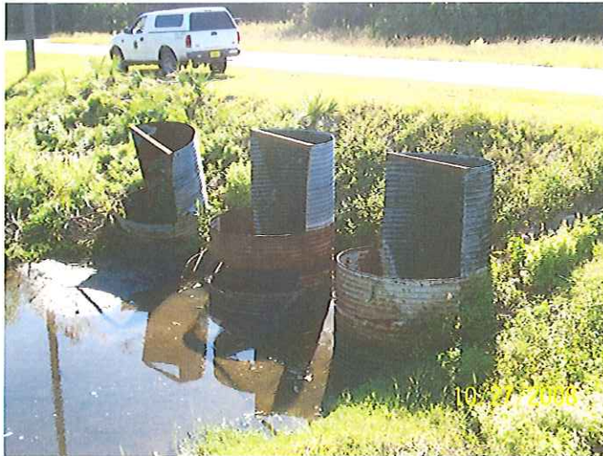
Old Corroded Water Control Structure #503 on Apollo Waterway
