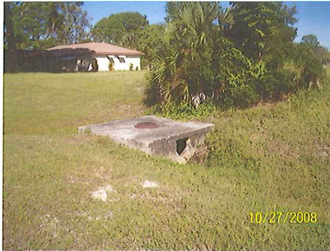
Old Water Control Structure #501 Discharging into Cheshire Waterway – 60” metal pipe connect to this concrete structure is corroded under Chancellor Blvd
