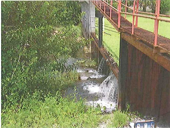
Old Water Control Structure #109 on Cocoplum Waterway with corroded metal weirs and 6 corroded gates. Note water pouring through large holes in the corroded metal weirs.
